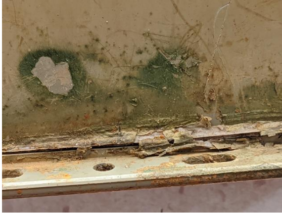
Figure 6: Flaking Near Well Riser
